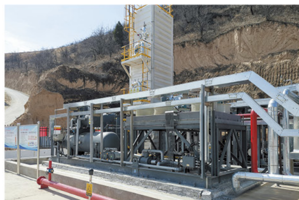
MRC compressor unit for 30,000 m 3 natural gas liquefaction
