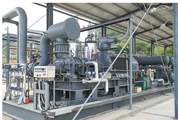
100,000m 3 natural gas liquefied water-cooled MRC unit
