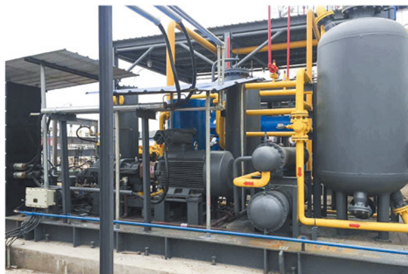
BOG compressor unit
