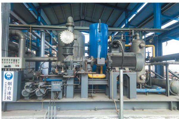
Flare gas recovery unit
