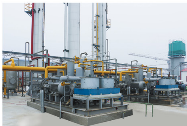
Biogas booster unit
