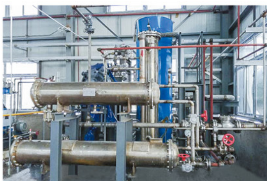
H 2 S Compressor unit
