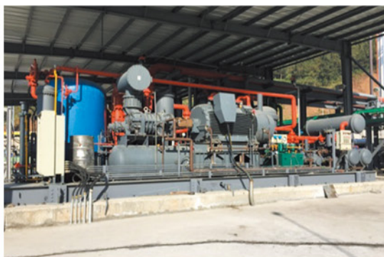
Nitrogen screw compressor unit for gas based LNG project
