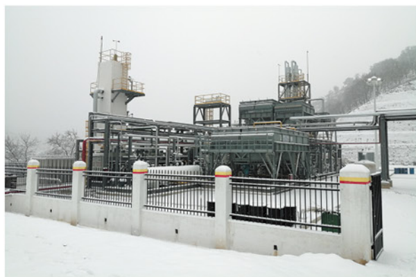
60,000m 3 natural gas liquefaction MRC unit
