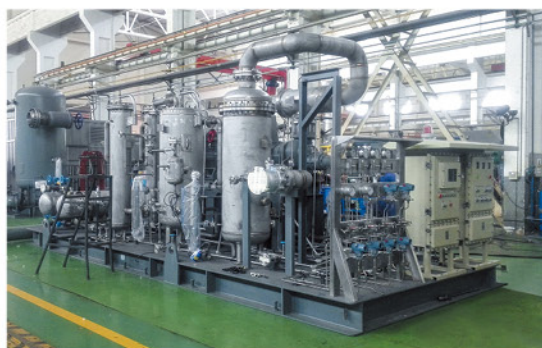
60t/h sour water stripping unit ammonia compressor unit project
