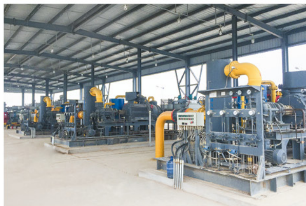
Coal bed gas compressor unit
