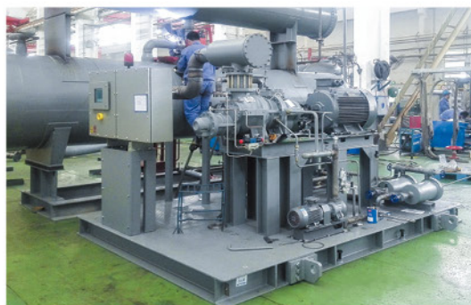
Sulfuric acid plant sulfur dioxide compressor unit
