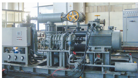
Ammonia booster unit of CO 2 liquefaction project
