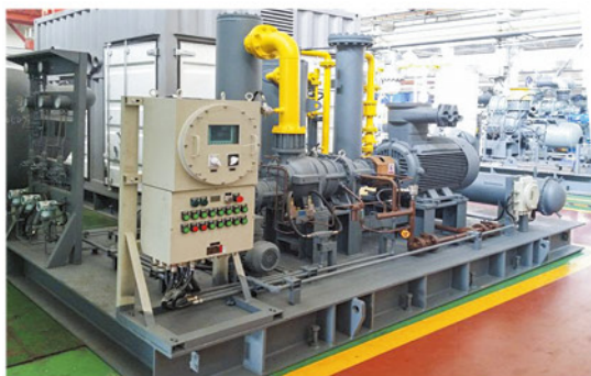
Sulfur dioxide compressor unit for smelting desulfurization liquid \text{SO}_2 project
