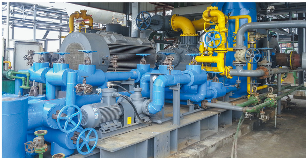
A C4S deep processing booster unit in Zhejiang
