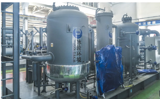
Coal chemical tail gas 100,000 tons food grade CO 2 pressurized liquefaction project
