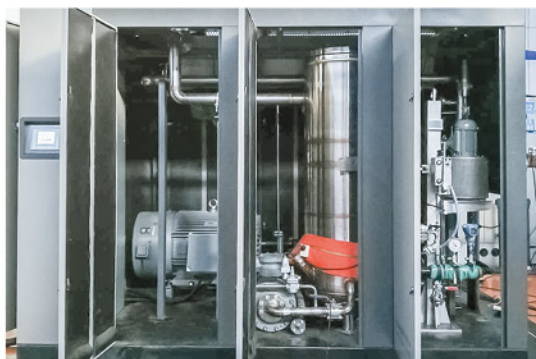
Helium screw compressor unit
