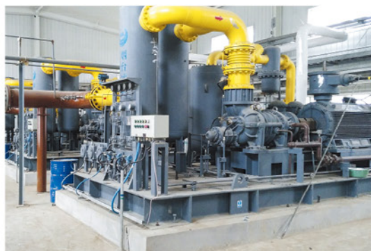
Vinyl chloride compressor unit for chlor alkali project
