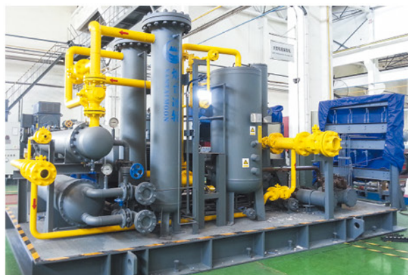
Natural gas compressor unit
