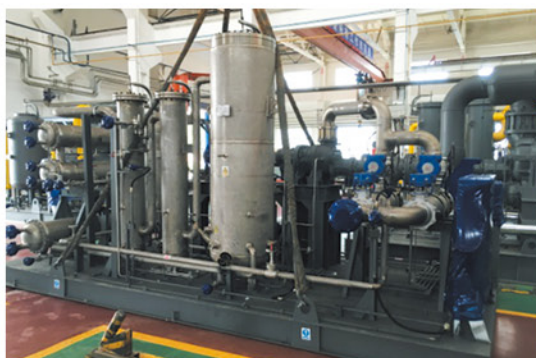
CS 2 compressor unit
