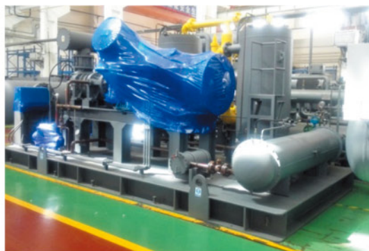
Nitrogen compressor unit of 200,000 ton/year mixed aromatization reconstruction project
