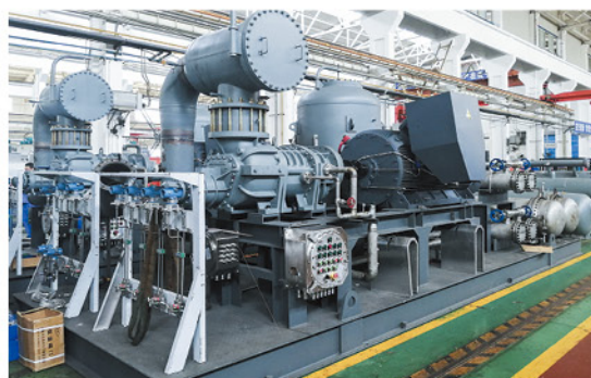
Ammonia compressor unit of acidic water stripping unit
