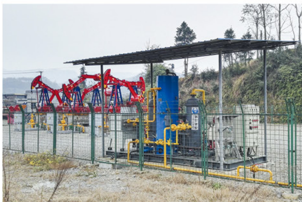
Oilfield gas production plant
